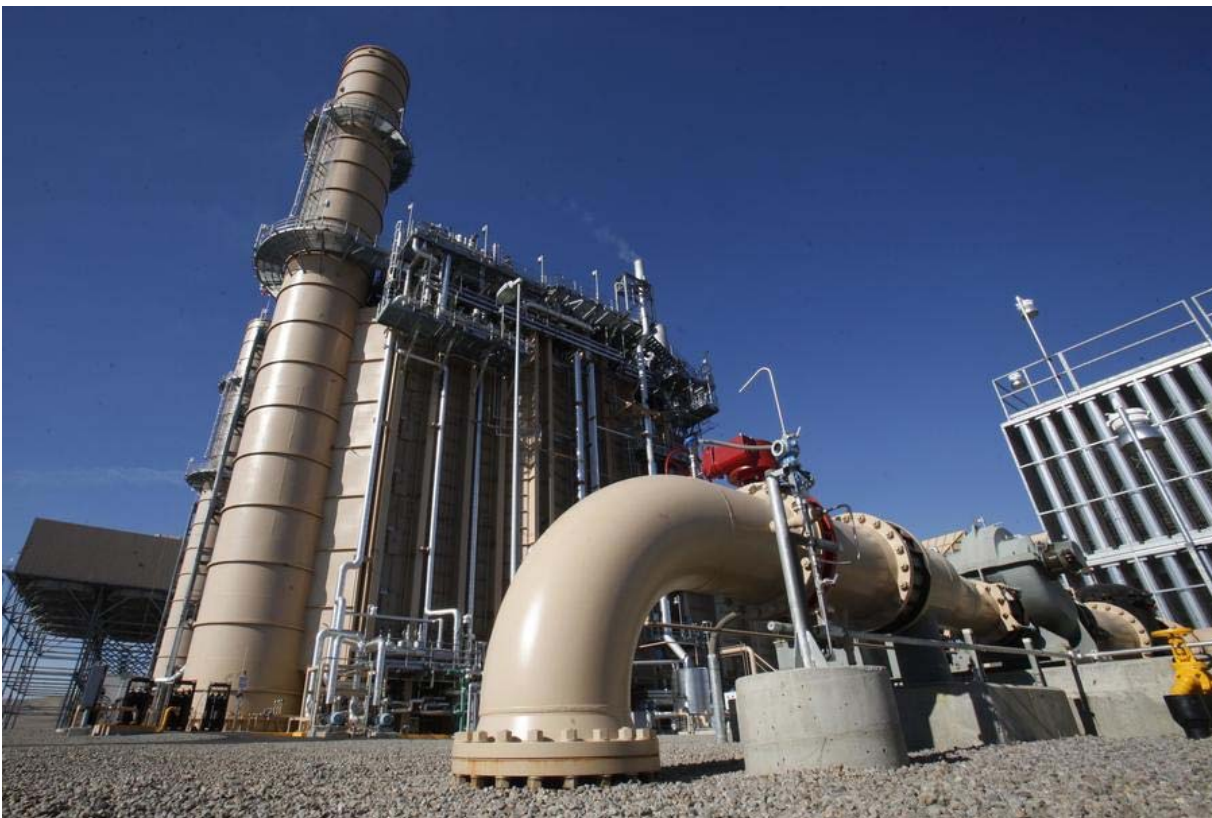
Pacific Gas & Electric's Colusa Generating Station has operated at well below its generating capacity — just 47% in its first five years. (Rich Pedroncelli / AP)
